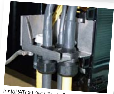
InstaPATCH 360 Trunk Cables attached to shelf mounted bracket
